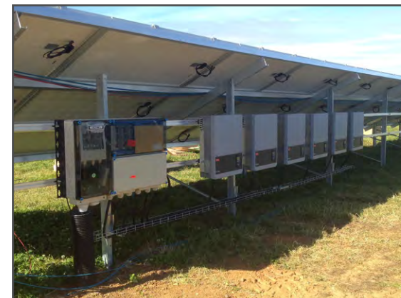
Plate 6 - Typical string-inverter units
